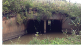
Storm Sewer under KIA Parkway
